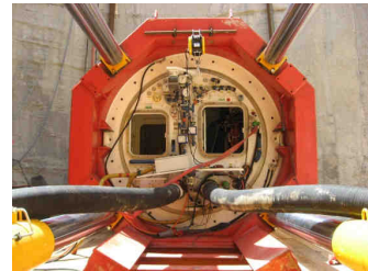
Integrated air lock chamber
