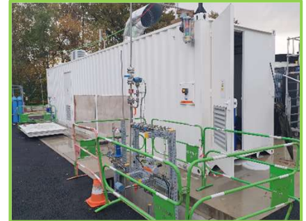
H 2 outlet lines to buffer tank
