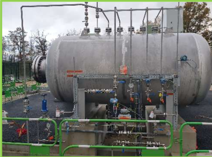
H2 Buffer Tank
